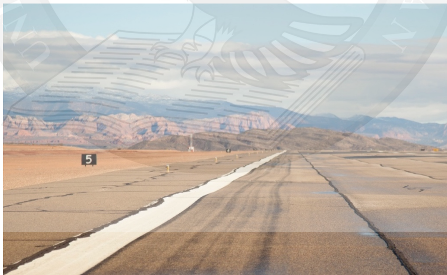
Gambar 1. 1 Pengembangan Expansive Soil Merusak Runway St. George Airport Sumber: https://www.thespectrum.com/story/news/2019/02/22/st-george-regional-airport-blue-clay-forcing-runway-closure/2919330002/
